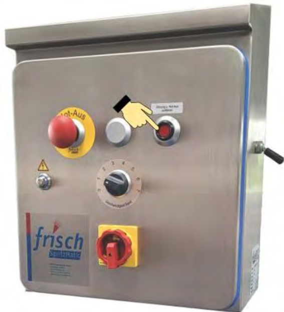
Figure 51: Acknowledging on the control panel
