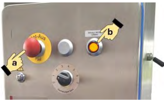
Figure 68: Emergency stop button on the control panel
