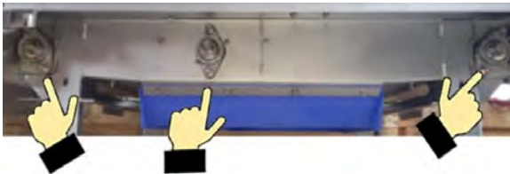
Figure 60: Bearing blocks on the belt conveyor
