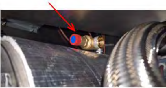
Figure 73: Heat exchanger safety valve
