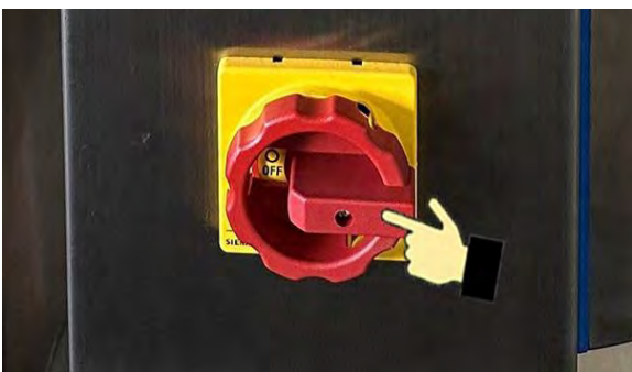
Figure 59: Switch off the main switch on the control panel
