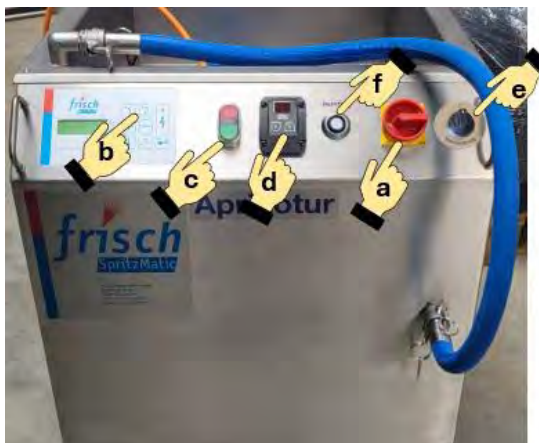
Figure 52: Switching on the heating machine with LWS
